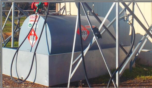
550 gallon tank in containment
