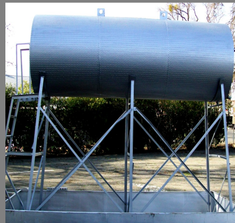
1,000 gallon tank on stand
