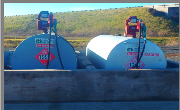
1,000 gallon tanks in containment
