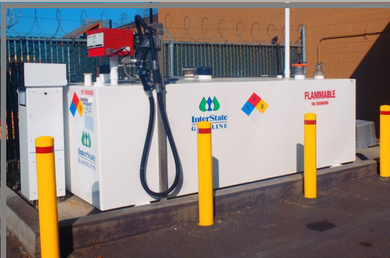
1,000 gallon vaulted tank with 110 volt pump
